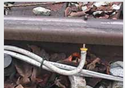
Application with track-side equipment through holes drilled in the rails.
