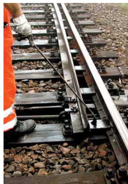
As in the past switch lubrication is mainly manual work.
